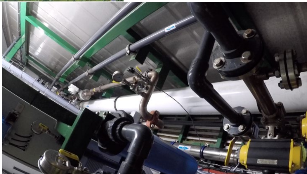
Station osmose inverse
